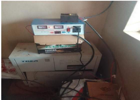
Inverter, charge control, and battery for solar system at Ngala CDSS
