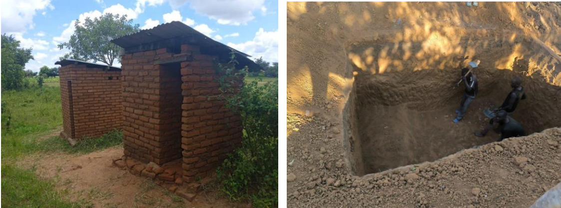
Left - Old latrines at Tchale Secondary School, Right - Workers digging a pit for the new latrines at Tchale Secondary during the month.
