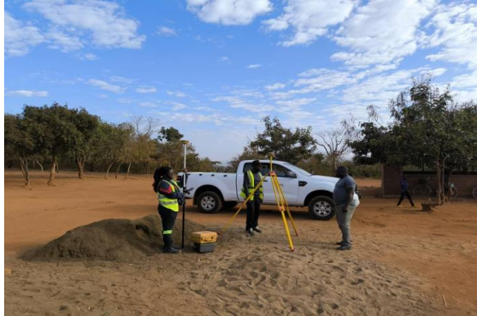
WASH Field Assistant Supervising the Land Surveying Exercise For The Piped Water Scheme At Kabuluzi School During The Month
