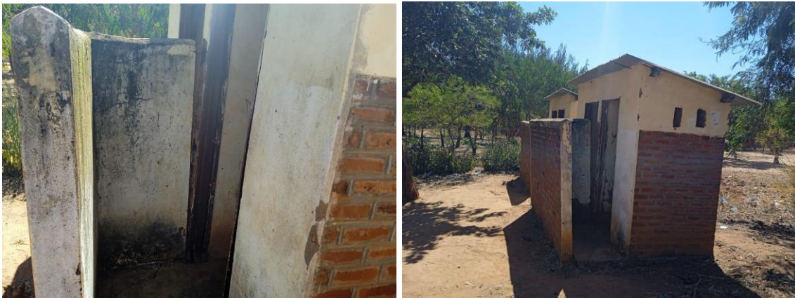
Photos of Boys' latrines at Nyagara Primary School which are in a bad state and are almost full
