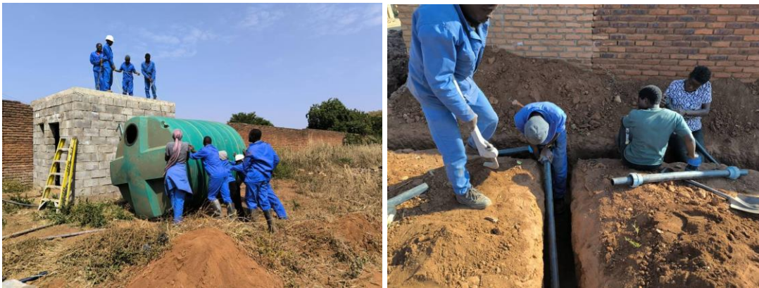
Left- Installation of a water tank for the Agroecology project, Right - Installation of a pipe networks
