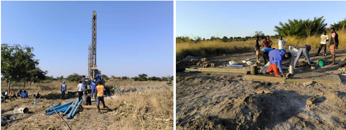
Left - Borehole drilling session during the month, Right - Construction of Aprons for the newly constructed boreholes during the month.
