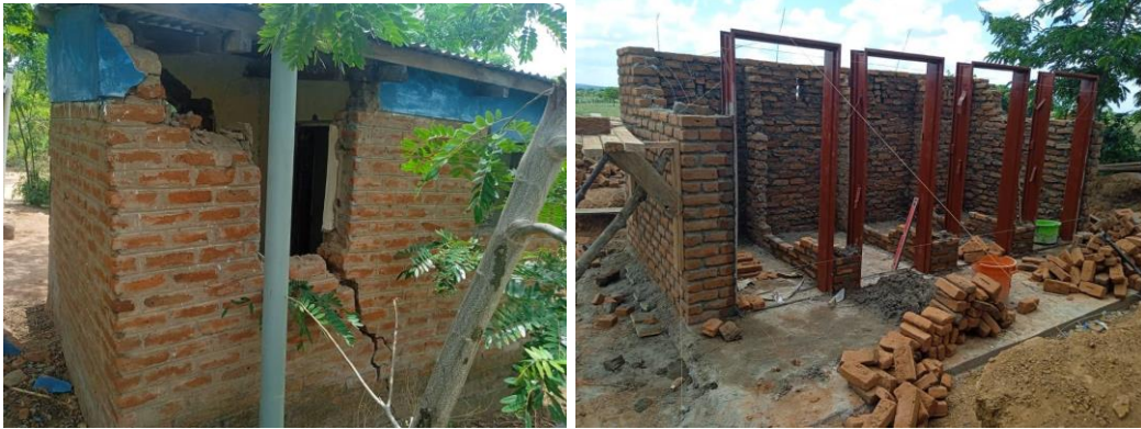
Left - Damaged boys' latrines at Mambala before OCA intervention, Right - Construction of boys' latrines at Mambala Primary School in progress.
