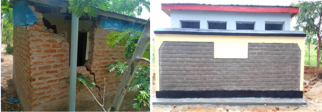
Left - Damaged boys' latrines at Mambala before OCA intervention, Right - Completed boys' latrines at Mambala Primary School.
