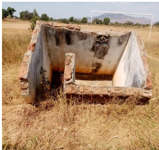
Damaged girls' latrines at Kalikulu before OCA intervention
