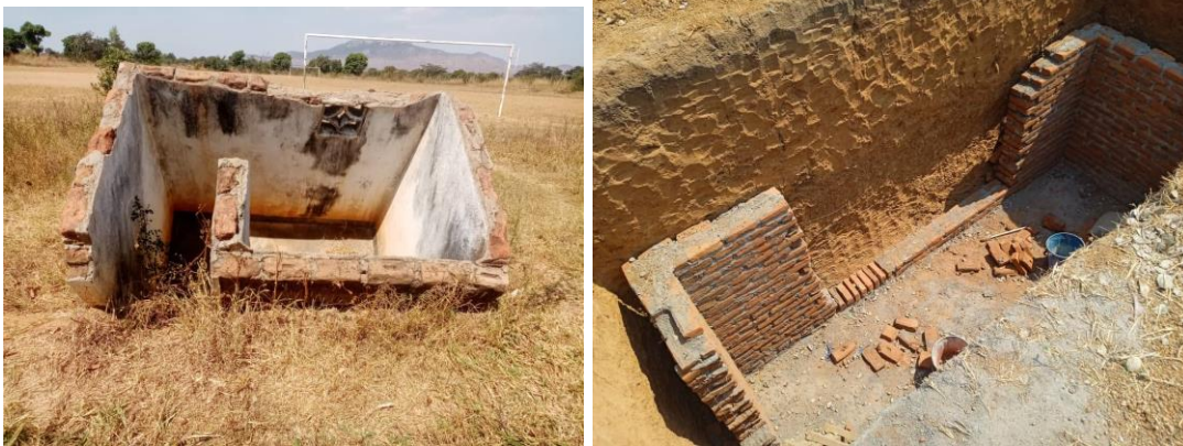
Left - Damaged girls' latrines at Kalikulu, Right- Construction of new girls' latrines at Kalikulu in progress
