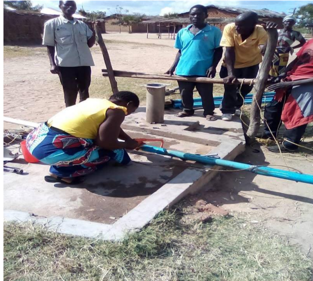
Afridev pump Area mechanic repairing raising main for a borehole in Mazinga village during the month
