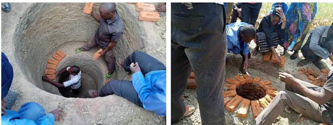
Left above- Early stages in the lining process of a corbelled latrine, Right above- Final stages in the lining process of a corbelled latrine
