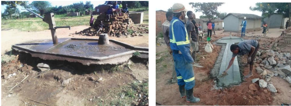
Left – Fulatila borehole with damaged apron before OCA intervention, Right - Borehole rehabilitation in progress in Fulatila village
