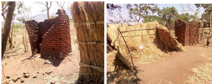
Figure 5: Images depicting the dilapidated state of latrines at N'dinga primary school
