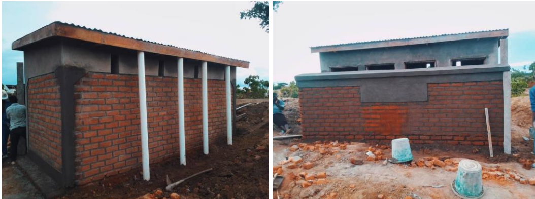
Rear and front view of a boys' latrine during construction in the month
