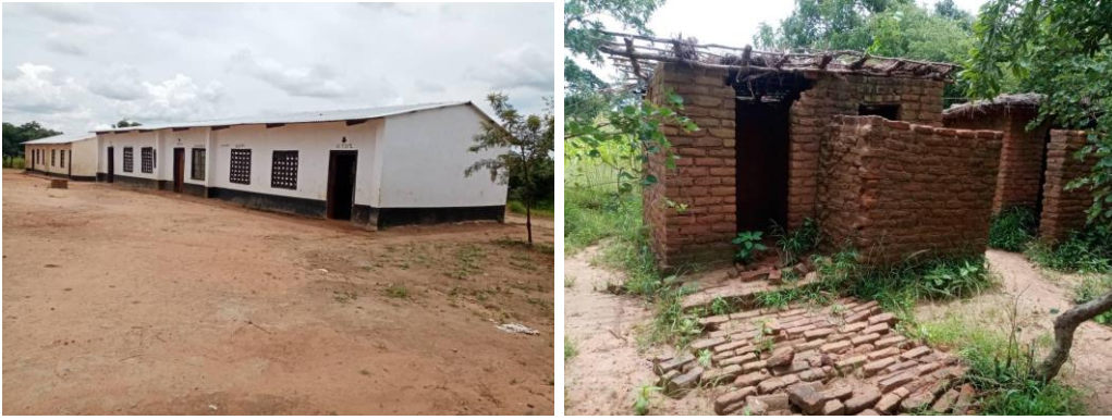
Left - Nambola primary school classrooms, Right - Current status of pit latrines at Nambola primary school
