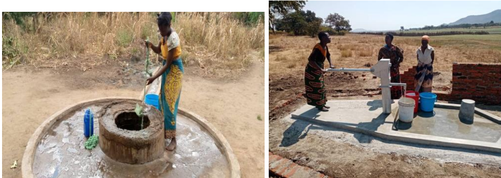
Left – Old water source in Nambela village, right – New water point constructed by OCA in Nambela village
