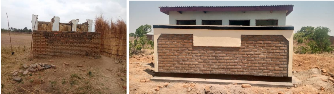
Left - Old dilapidated pit latrines at Madzo primary school, Right - New girls latrines constructed by OCA at Madzo primary school before handover
