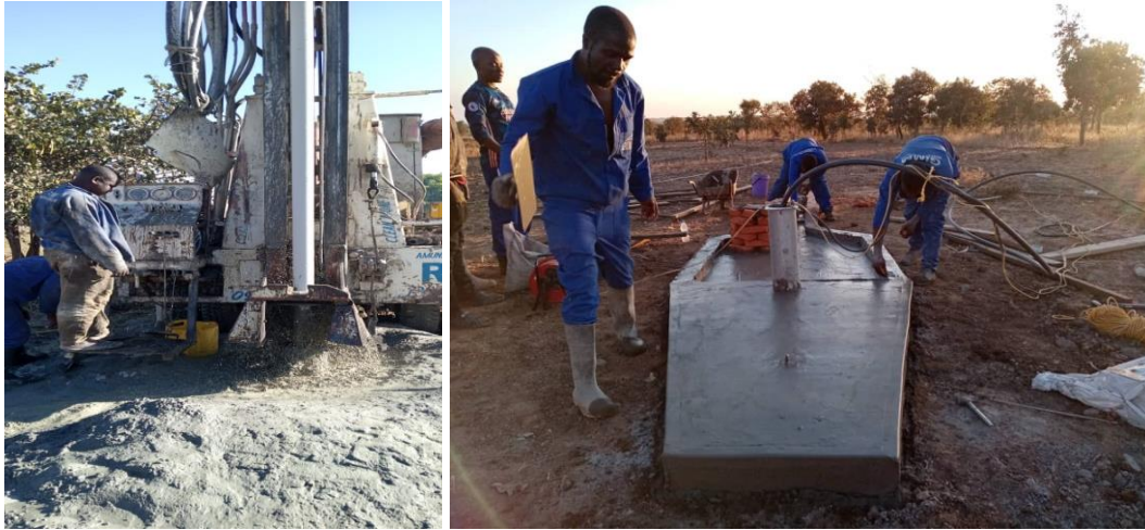
Left – Borehole drilling at Chinkha village, Right – Borehole civil works in Soko village before handover
