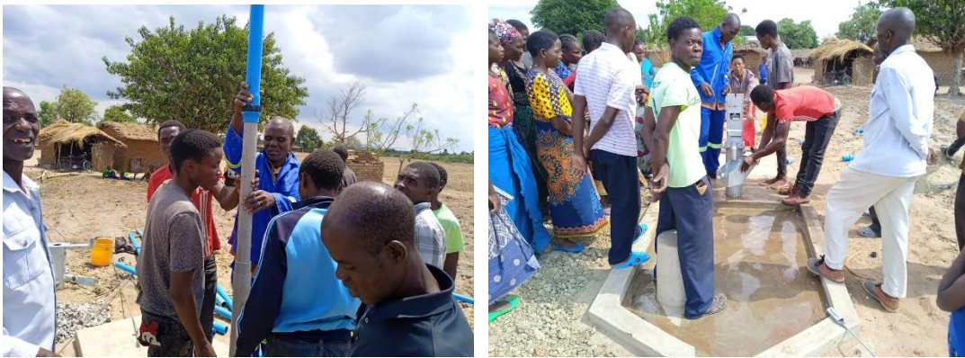
Left- Pump repair session at Kasinja village during the month, Right – Kasinja borehole now fully functional following a repair session
