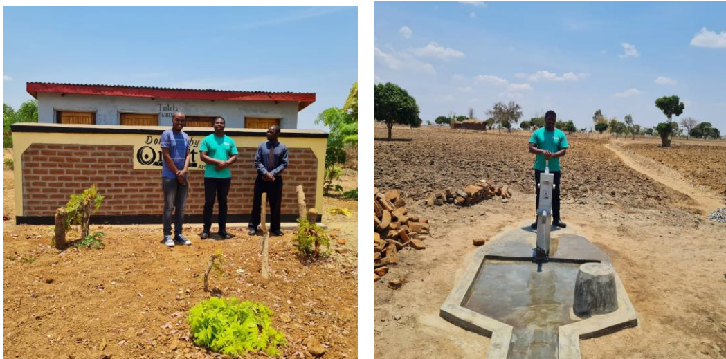
Left – Newly constructed latrines at Nambola school during the CD's visit, right – New borehole drilled with support from OCA in Kam'phika village during the CD's visits
