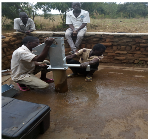
Image showing new pump head being installed and the community taking part
