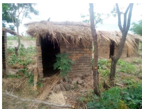
The top two images show the front and back views of the newly constructed latrine (before branding) and the below image show the old latrines at the school.
