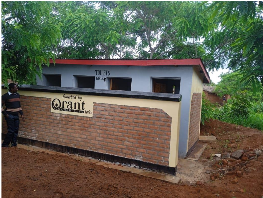
A new girls' latrine at Kapini primary school which is now in use
