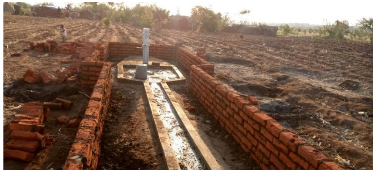
Completed borehole (not yet in use) and the community is building a fence using its resources
